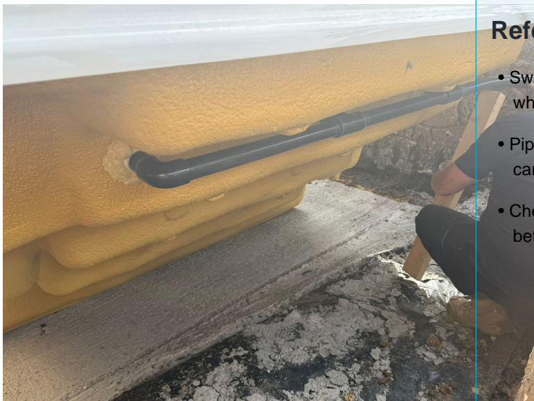
Reference photo: installed pipe route with bends and fittings.
